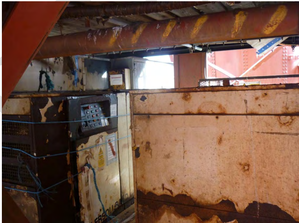
Compressor and interior of housing
