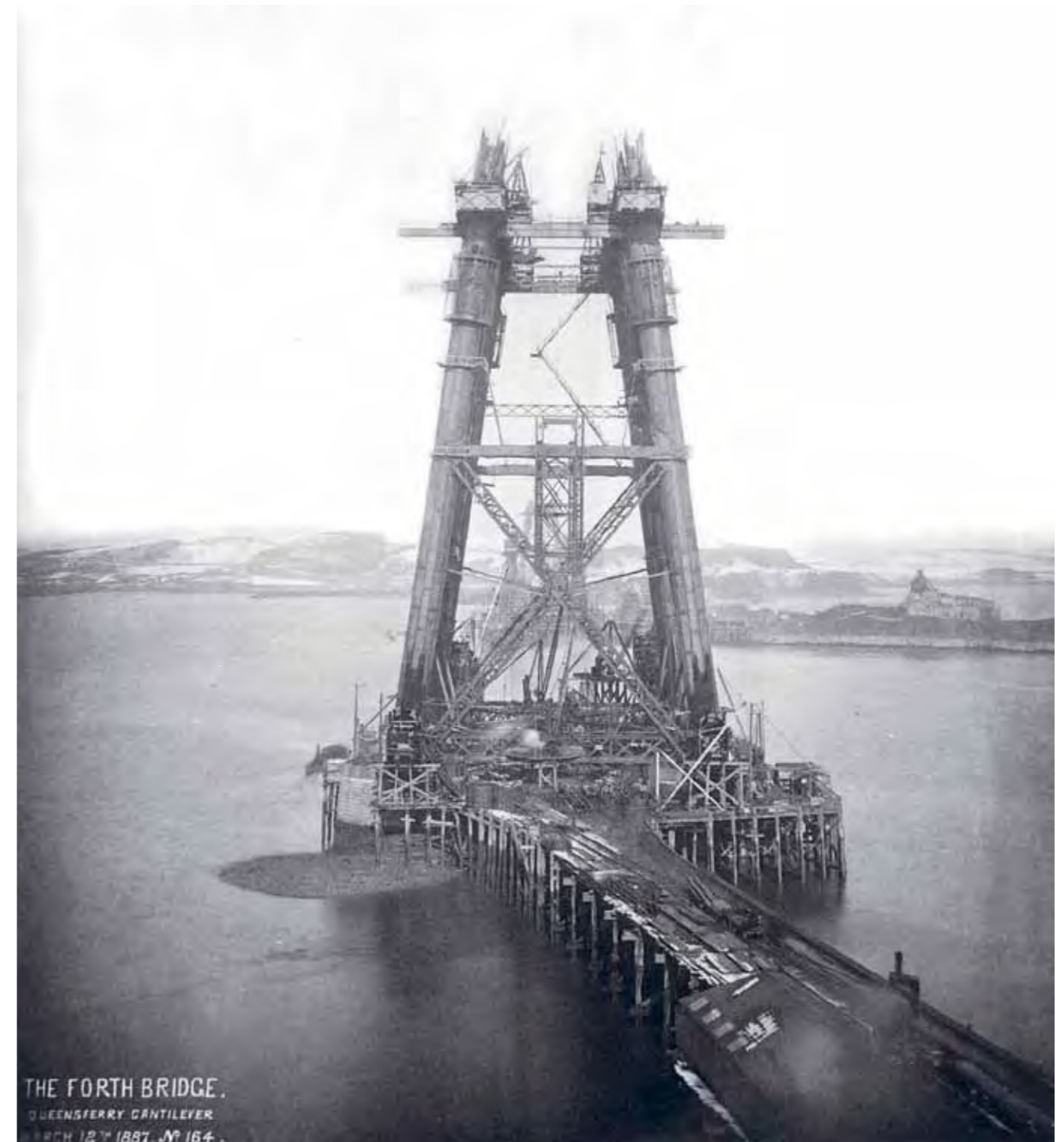
Photograph showing progress of the Queensferry main tower on 12 March 1887, (© Crown Copyright, National Records of Scotland).
